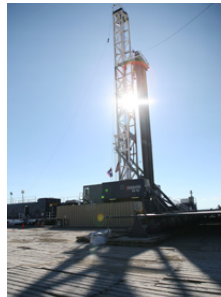
The raised platform used by Encana at some of its drill sites helps to protect the underlying landscape. (Credit: Abrahm Lustgarten/ProPublica)
