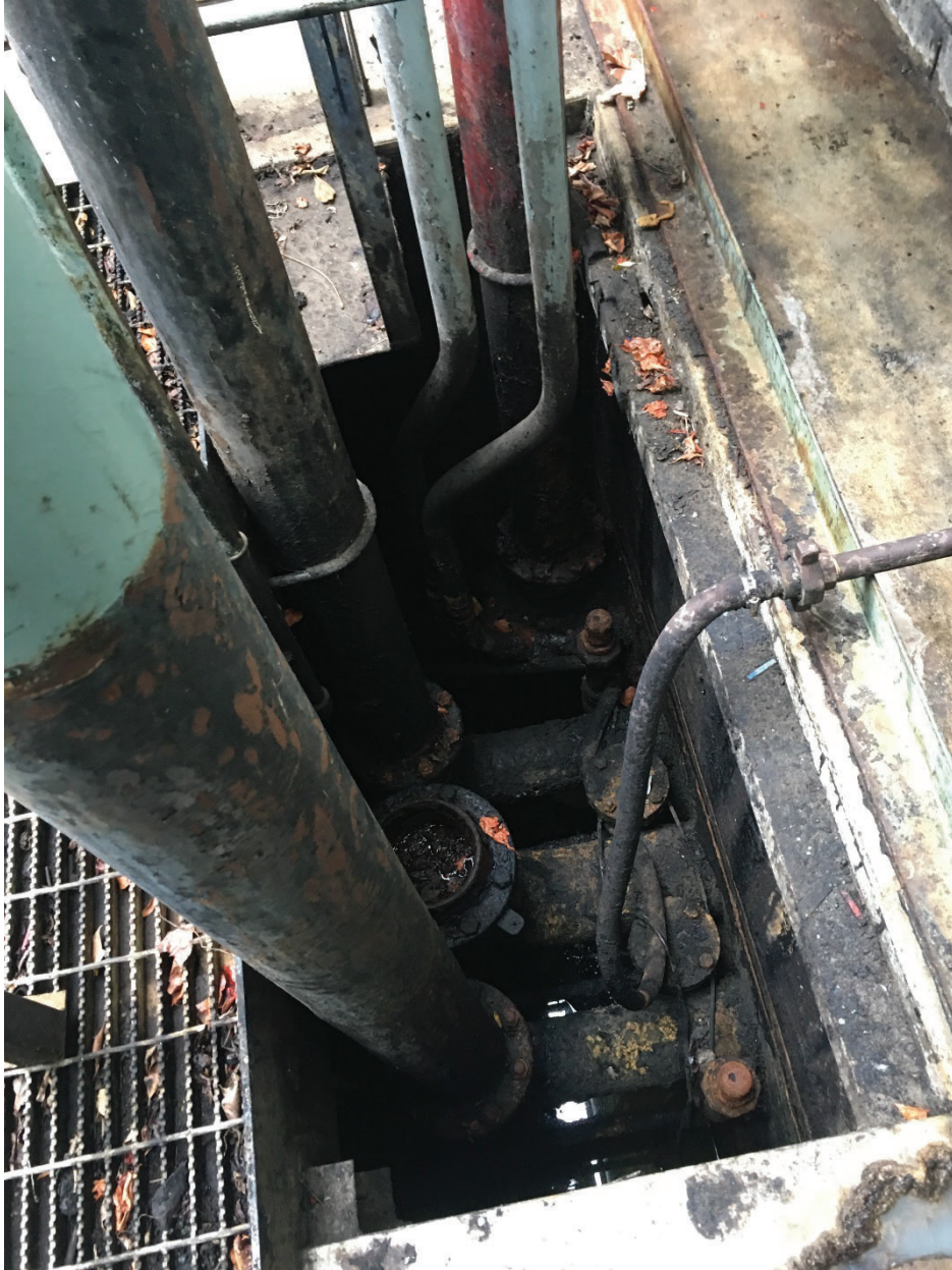
Figure 10. This photo shows the out of service lines entering the cement to run underground to the production facility. The two 6-inch lines were still connected to the pressurized pipeline system but isolated with a "slip blind" that failed.
