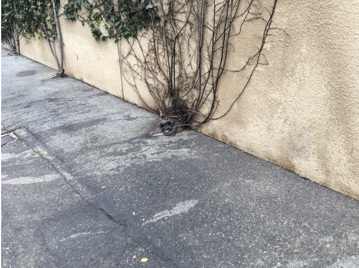
Figure 6. The fluid was extruded through the joint where the building wall met with the asphalt alley. The area shown here was the main location of leaking with minor leaks further east and west in the photo. The area which had leaks was approximately 10 feet in length.
