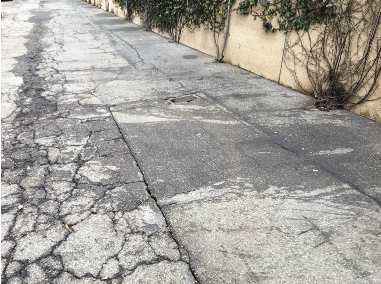
Figure 3. Staining shows point source with most discharge as well as lateral extent into the alley
