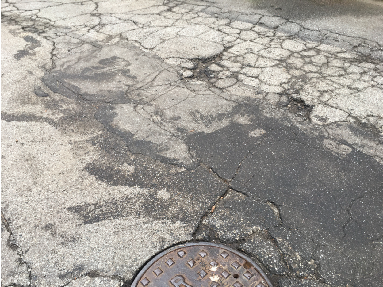
Figure 5. shows leaked fluid migration extent
