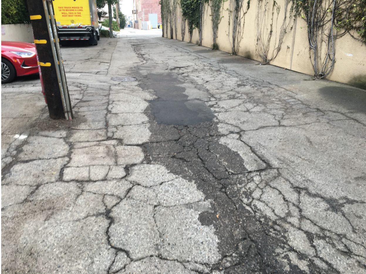
Figure 4. Shows areal extent of leaked fluid migration
