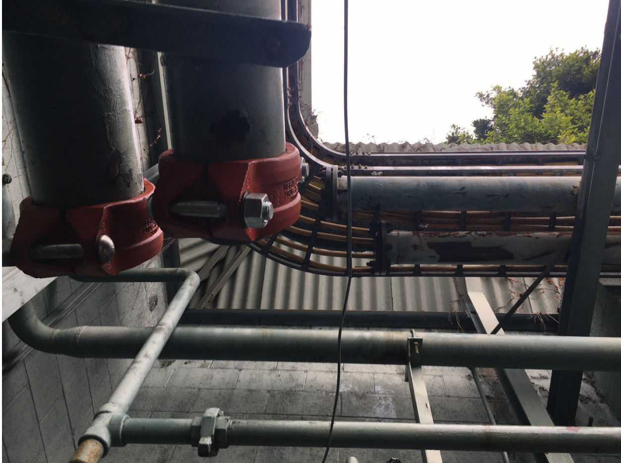
Figure 11. The photo shows the out of service pipelines with red caps having been disconnected from the horizontal pipelines that are still under pressure. At the time of the leak, these two ends were connected and the out of service segment was isolated from pressure with the use of a “blind slip” that was found to be corroded to the point of leaking.
